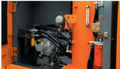
Grouped remote filters and inspection points
